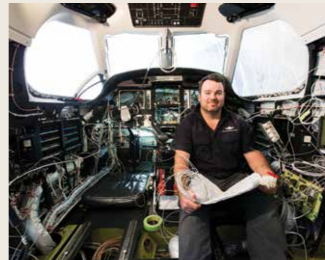
Apprentice engineer Brenton Kenneally at work on the interior refit of 'November'.
